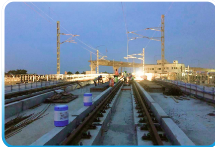
SIEMENS - Metro Depot Ingeniery for life
