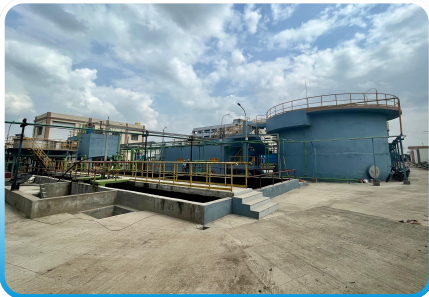
Haldiram's Haldiram's - STP/ETP
